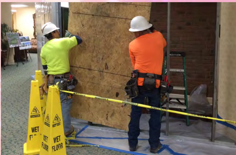
And so it begins!! The work on the new Kirby Bistro has started and we can't wait to see it develop
